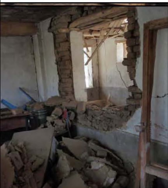
Blast damage Do Abe Coord Centre IED
