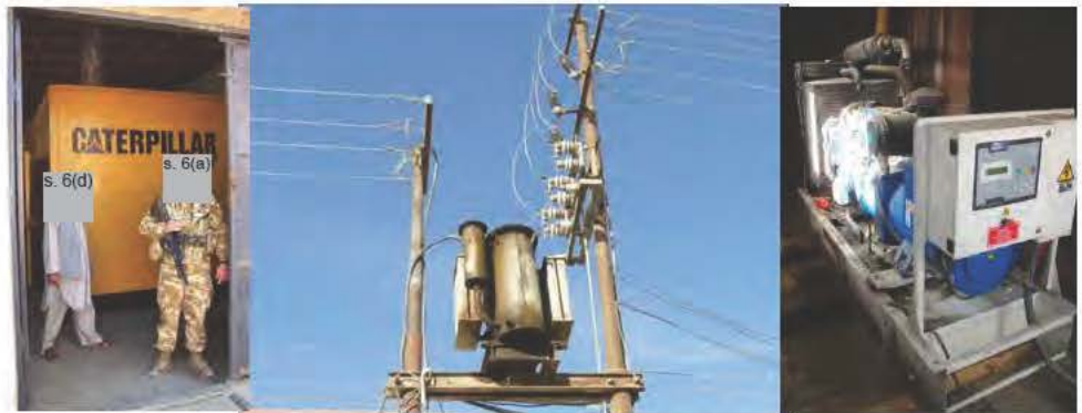
Bamyan's two generators are relatively new but have had no diesel for 9 months.
