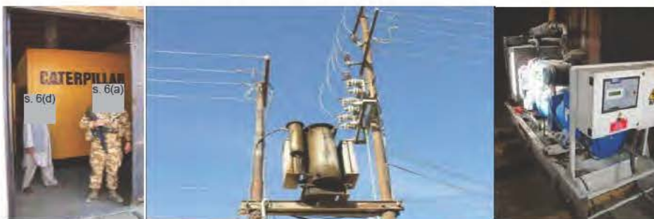
Bamyan's two generators are relatively new but have had no diesel for 9 months.
